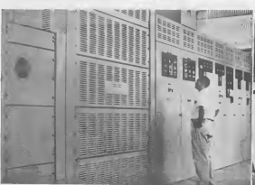
THE NEW switchgear is compact and entirely en- closed. E SWITCHCHAN nobo ta compacto y henteramento di J. Lymer, Mechanical-Electrical, stands in cerra. J. Lymer, Mechanical-Electrical, ta pará dnaní frowd di new stub 10 worked on by R. Brown and M. stab 10 nobo ariba coal ta traha R. Brown y M. Emanuels, handa drechi, Mechanical-Electrical.
